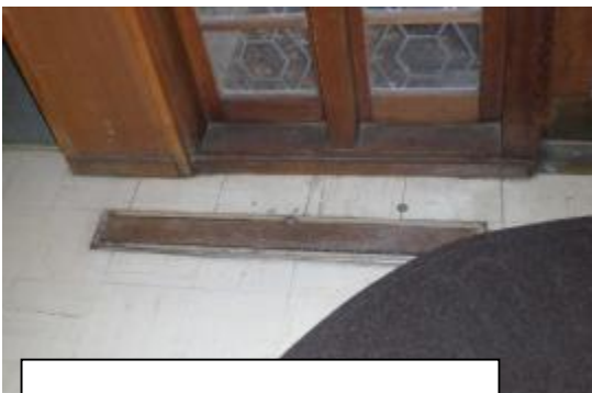
Figure 13 – Blocked off vent in Lounge area.
