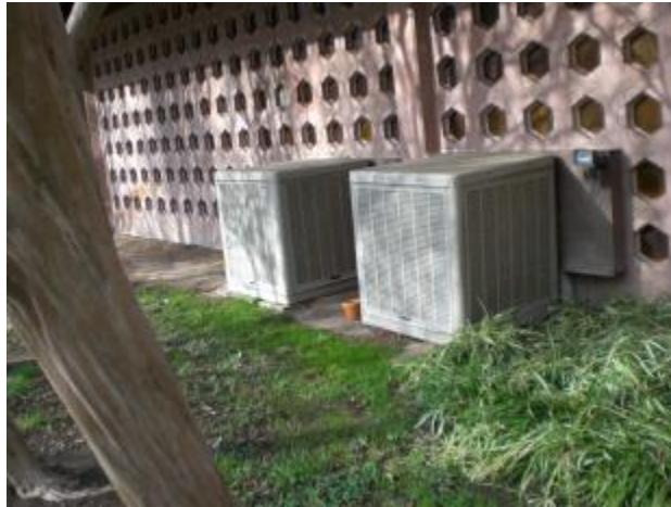
Figure 15 –Evaporative Coolers for Main Hall.
