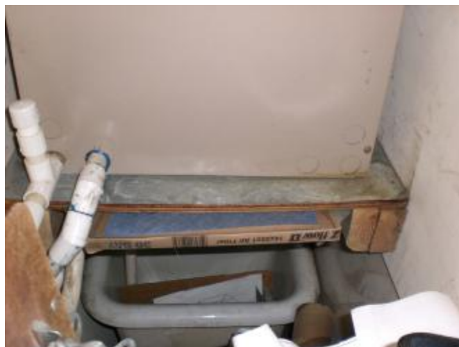
Figure 17- Filter and tub at intake of AC unit.
