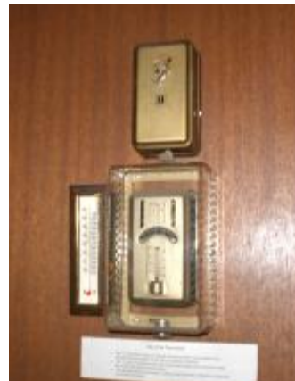
Figure 14 – Thermostat for large heating system in Main Building.
