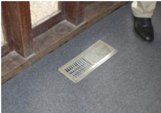
Figure 11 – Typical perimeter vent in office space.
