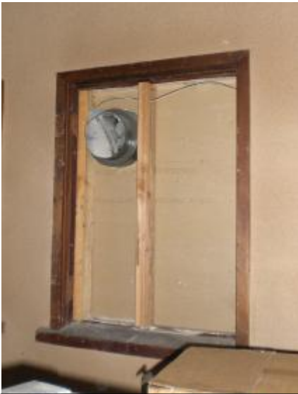
Figure 18 – Exhaust fan from bathroom to loading bay.
