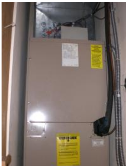
Figure 16 - Air conditioning unit for offices and library.
