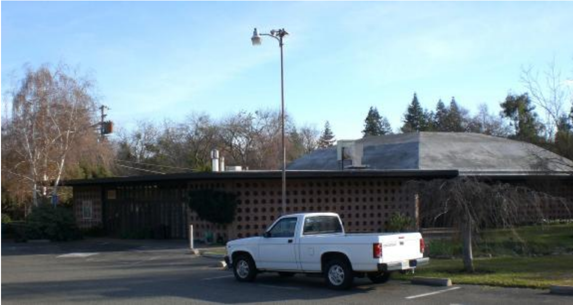
Figure 4- Flat roof on office/kitchen/library portion of Main Building. Dome roof over Main Hall.
