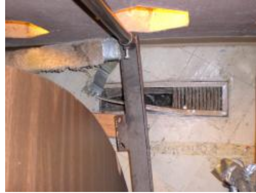
Figure 10 – Damaged vent in table storage area.
