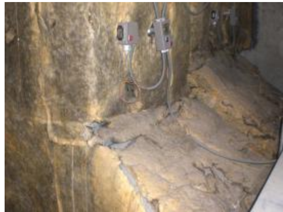
Figure 12 – Supply ducts for furnace with analog sensors and controls.
