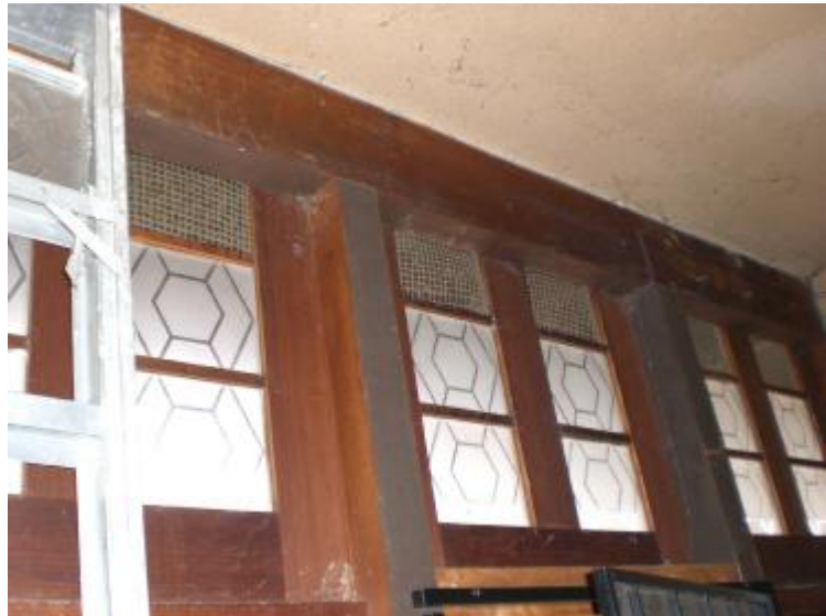
Figure 19 – Openings for fresh air for main furnace and relief for bathroom ventilation fans.
